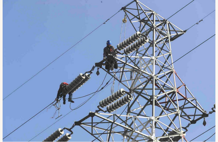
High-voltage lines: thick, bare aluminium – why?
